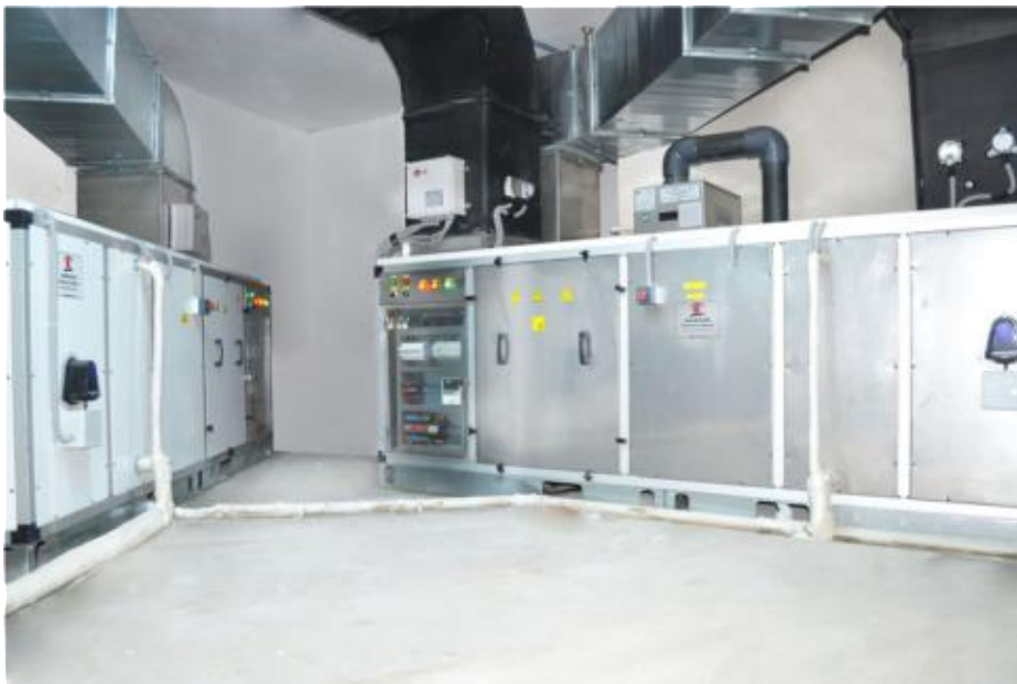
Hygiene AHU in the hospital
