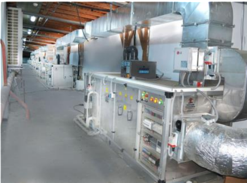
Hygiene AHU in the hospital
